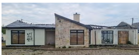
Photo above displays bulletproof windows & property damage from arson attack
